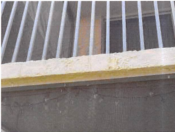
6.j Spalling in small areas.
