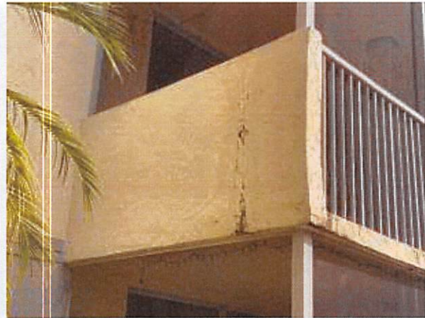
6.i Cracks in small areas
