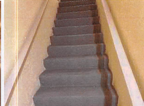
7.b.3 Stairs in fair condition
