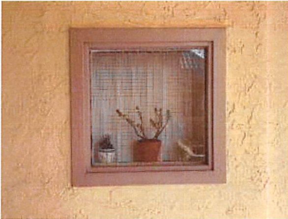
10. Windows in fair condition
