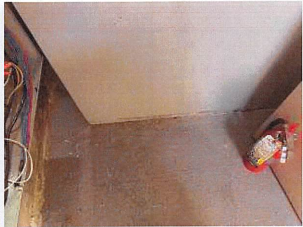
8.f Elevator machine room
