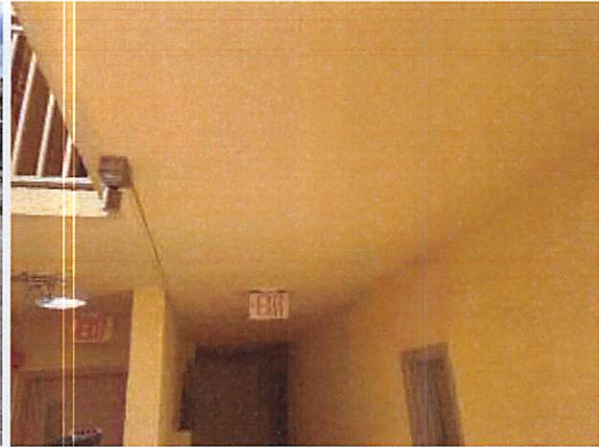
7.b.1 Floor system in fair condition
