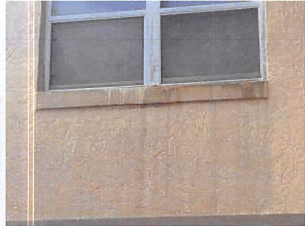
5.c Hairline cracks on stucco
