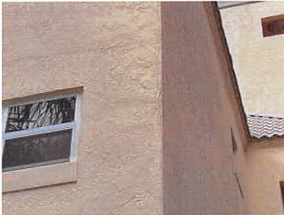
5.d Fine cracks on walls
