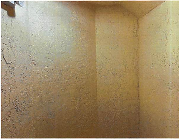
6.h Interior paint in fair
