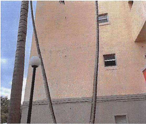
6.j Spalling in small areas.
