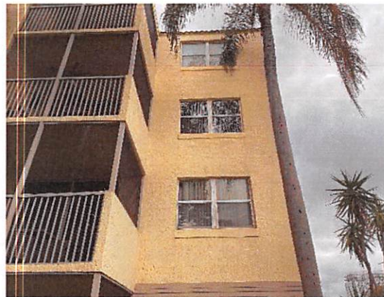
5.c Hairline cracks on stucco
