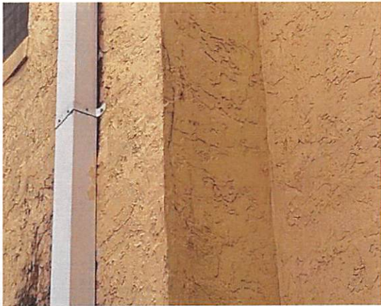
5.d Hairline cracks on walls
