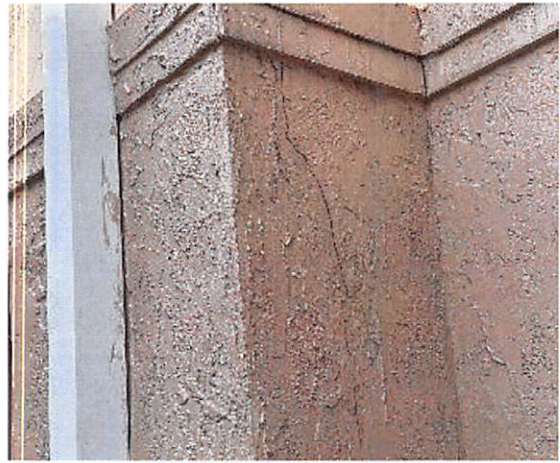
6.i Cracks in small areas
